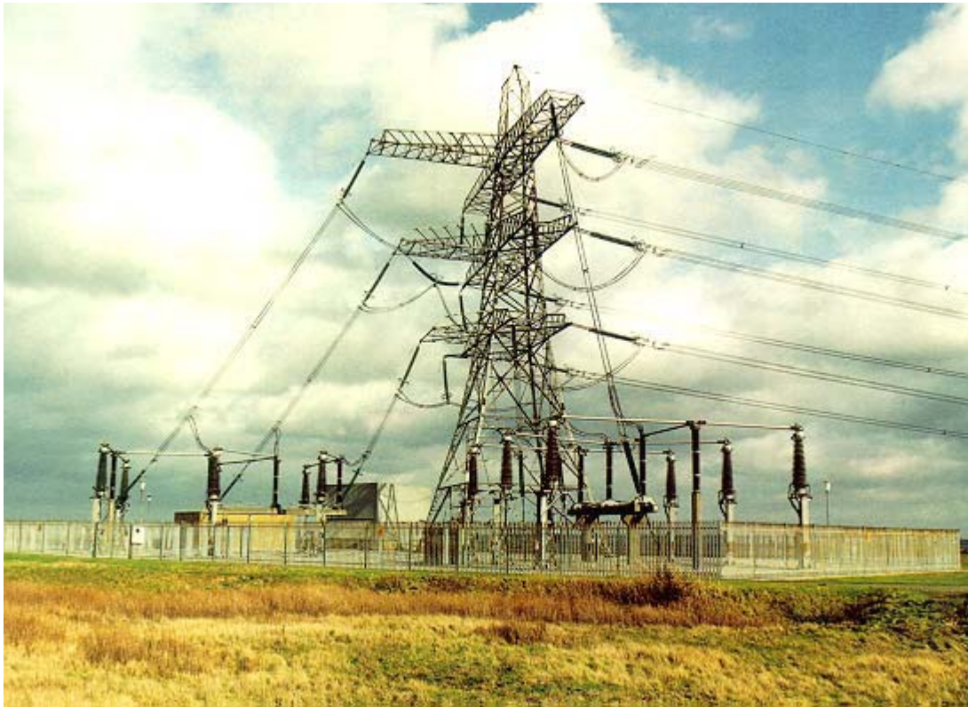
Figure 3.18: 400 kV transition compound
