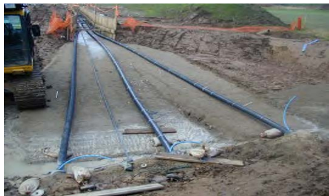
Cable spacing increased as cables enter ducts
